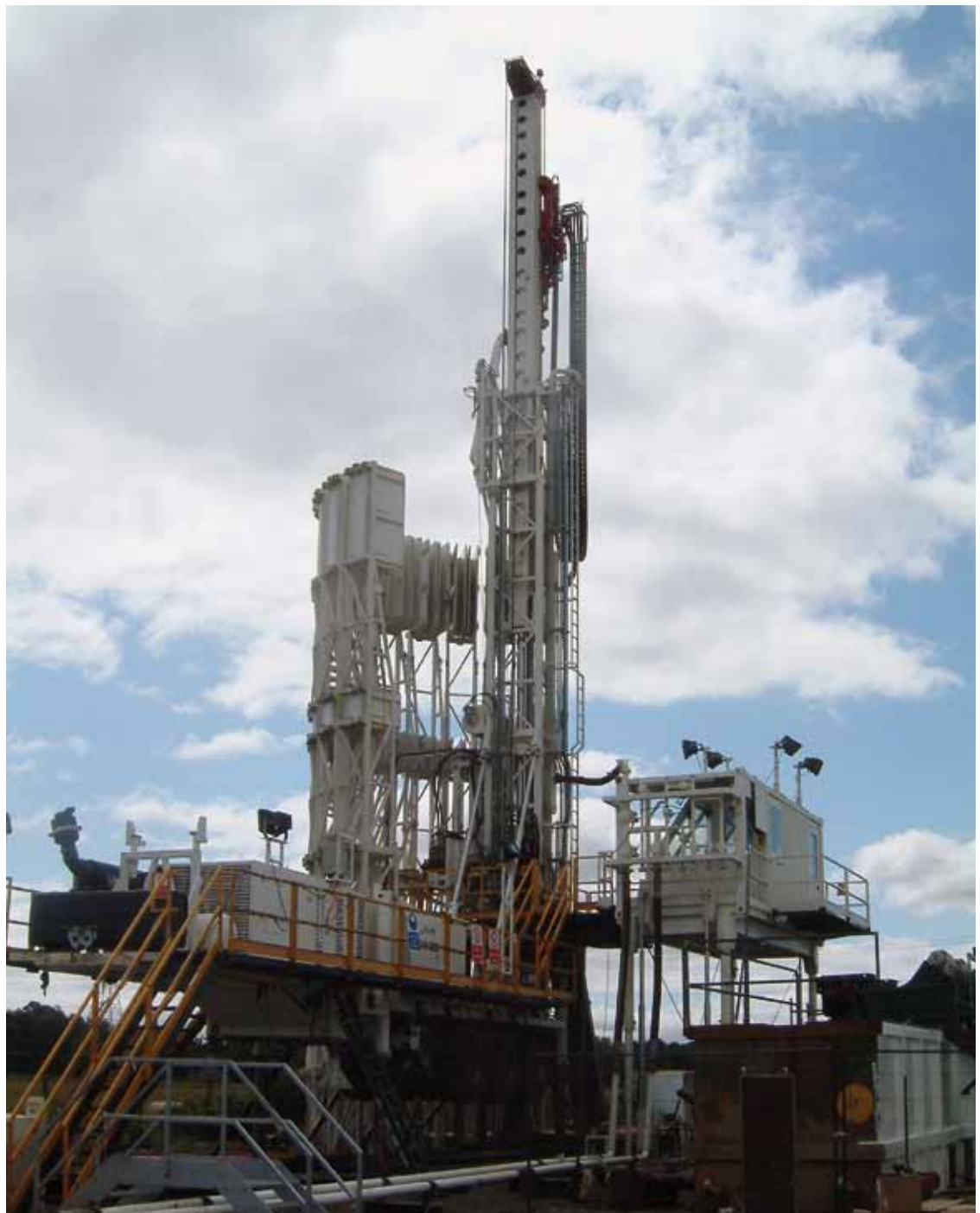
A modern drilling rig equipped for long-reach directional drilling in deep coal seams. The semi-circular rack behind the rig mast is an automated drill-pipe carousel © Paul Younger
